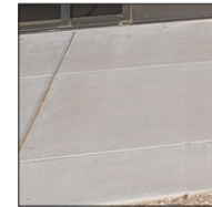
MATERIAL M8 POURED IN PLACE CONCRETE STANDARD GRAY CONCRETE SIDEWALKS AND CURBS
