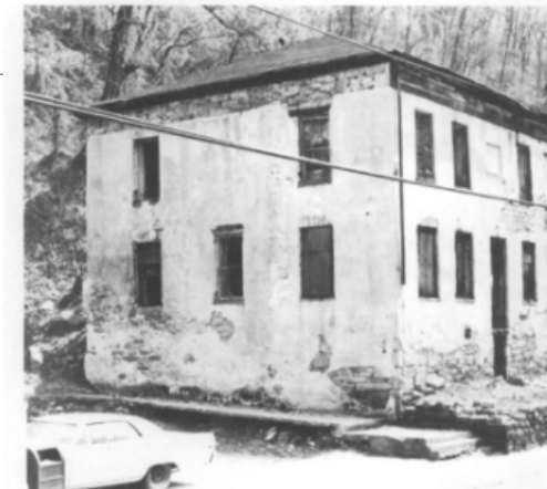
Fig. 7. Patches of stucco have fallen off this derelict 19th century structure exposing the rough-cut local stone substrate. The missing wood entablature on the side and the rough wood lintel now exposed above a second-floor window, offer clues that the building was stuccoed originally. Photo: National Park Service Files.
