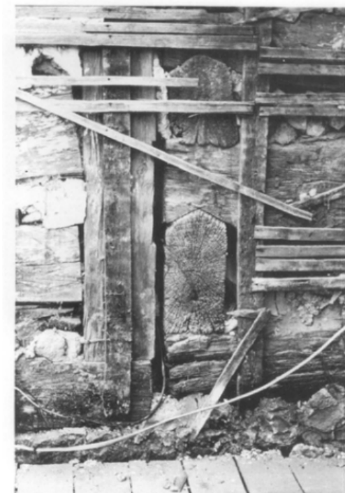
Fig. 8. Removal of deteriorated stucco in preparation for stucco repair on this late-18th century log house in Middleway, West Virginia, reveals that the stucco was applied to hand-riven wood lath nailed over vertical wood strips attached to the logs. Photo: Anne Grimmer.
