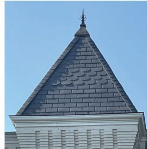
Figure 10. Polymer slates offer a choice of shapes but not sizes, limiting their ability to achieve a good visual match for some historic slate. With the size of the polymer slates (right) being nearly twice that of the historic slates (left), the scale of the entire feature is incompatibly altered. The molded edges of this material, which contribute to its ability to replicate slate, would be lost if each shingle was resized by cutting. Photo: John Sandor, NPS.
