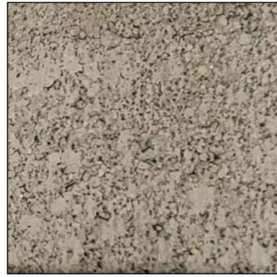
B CMU: FINISH: PRECISION MFG: SUPERLITE BLOCK COLOR: "HUNTINGTON GRAY-NW GRAY" WITH DARK GRAY RACKED GROUT
