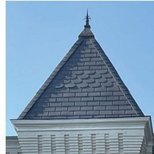
Figure 10. Polymer slates offer a choice of shapes but not sizes, limiting their ability to achieve a good visual match for some historic slate. With the size of the polymer slates (right) being nearly twice that of the historic slates (left), the scale of the entire feature is incompatibly altered. The molded edges of this material, which contribute to its ability to replicate slate, would be lost if each shingle was resized by cutting. Photo: John Sandor, NPS.
