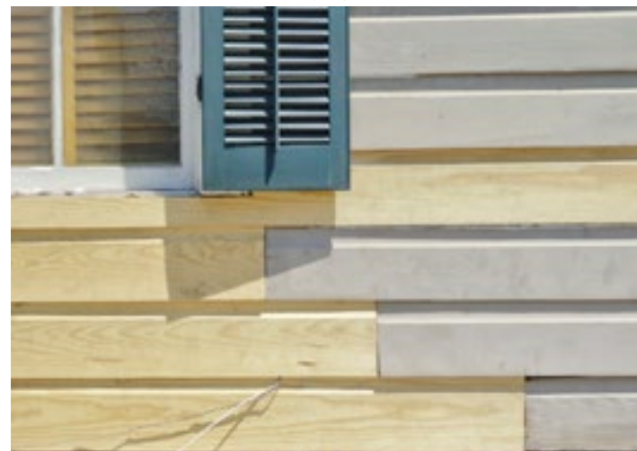
The Dutchman repair method allows for the installation of new wood while preserving the historic wood.
