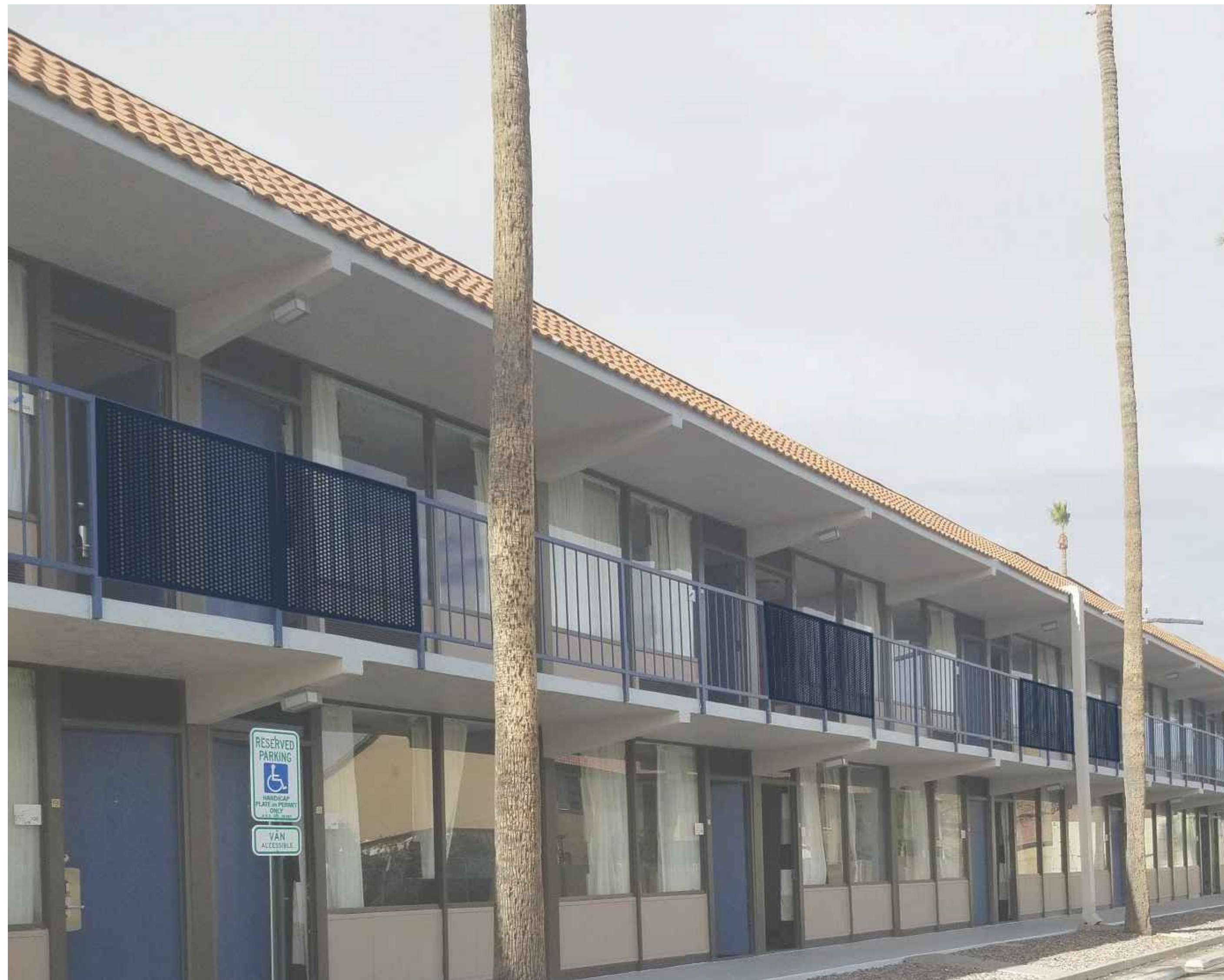
ARCHITECTURAL SCREEN MATERIAL PLACED ON EXISTING 2ND STORY HANDRAILS ON THE RESIDENTIAL BUILDINGS. FINAL PAINT COLOR TO BE COORDINATED WITH ARCHITECTURAL COLOR PALETTE. SCREEN MATERIAL WILL MATCH MATERIALS USED AT ENTRY AND ON BUILDING 2.
