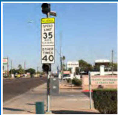
Communications Equipment & Programming Software for School Zone Flashers
