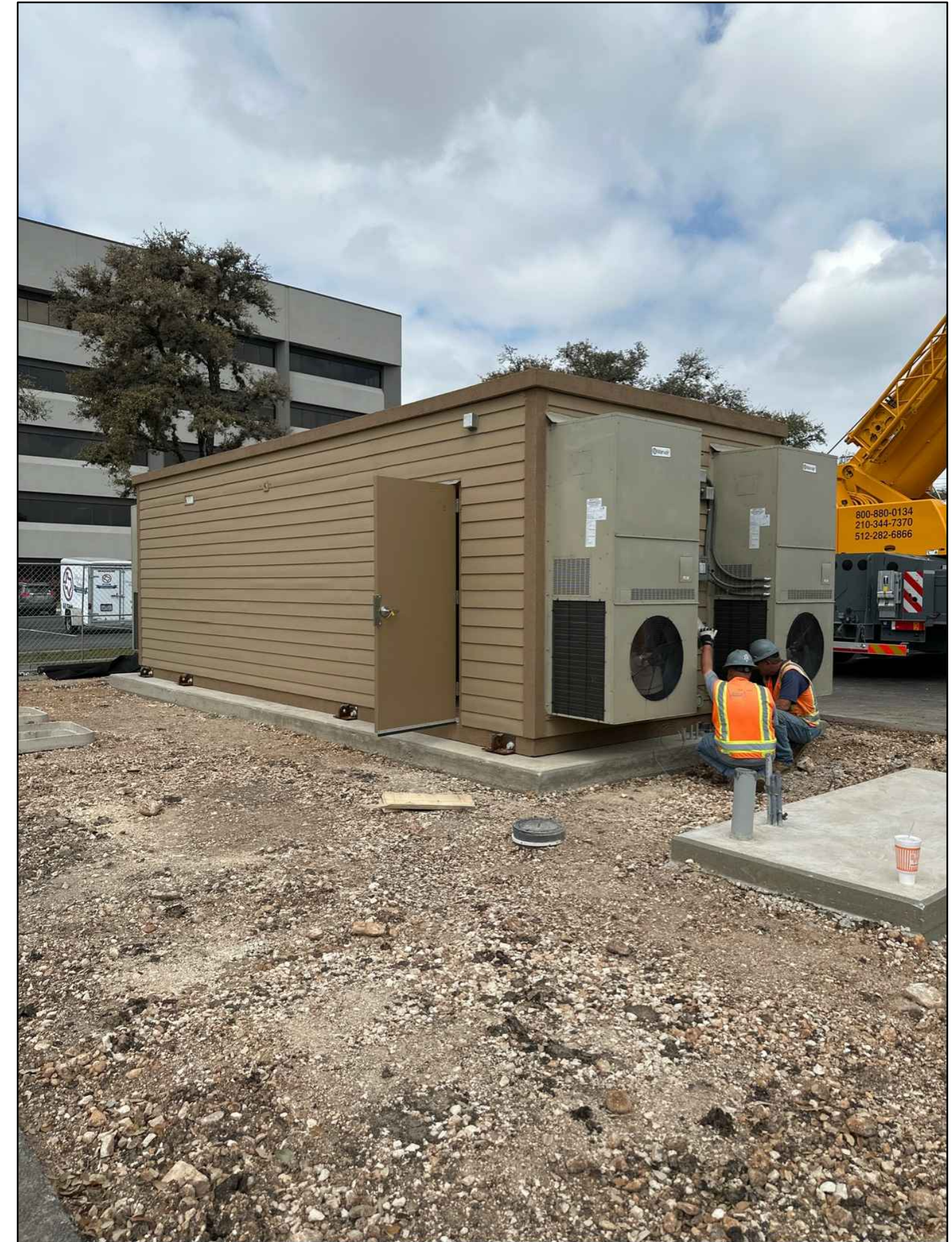
IMAGE OF EQUIPMENT SHELTER BUILDING
