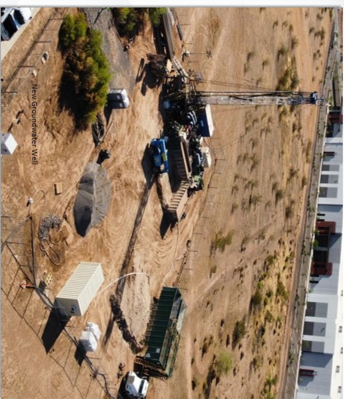
New Groundwater Well
