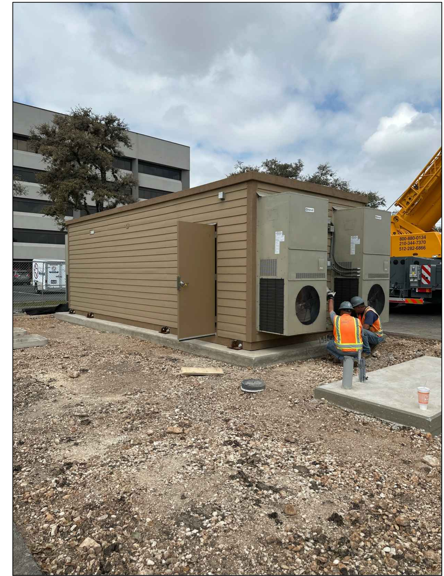
IMAGE OF EQUIPMENT SHELTER BUILDING
