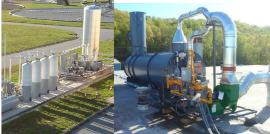
Figure 7. PSA RNG Upgrading Skid and Thermal Oxidizer
