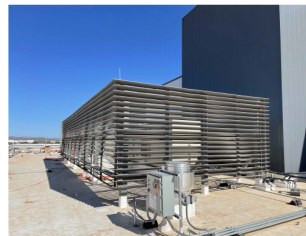
LOUVERED EQUIPMENT SCREEN
